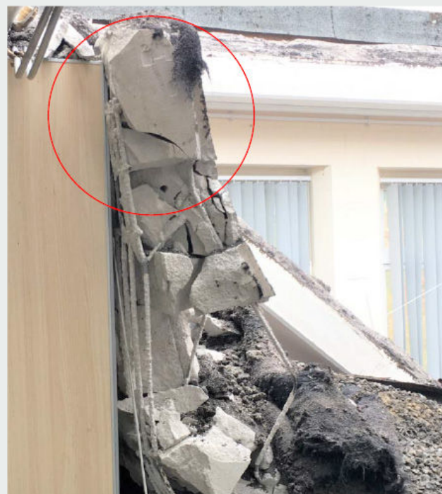
● Figure 1 The 2018 roof slab collapse
