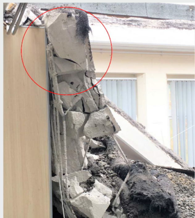
● Figure 1 The 2018 roof slab collapse
